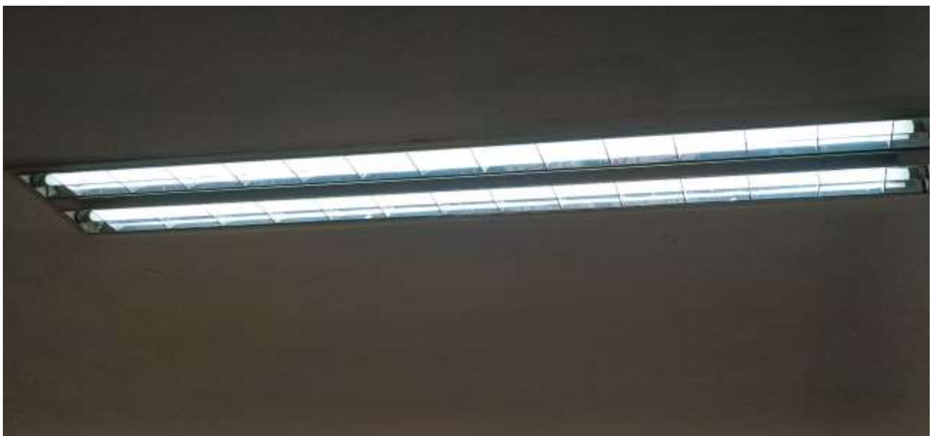
Fig.: 3.5 Electrical Equipments in Institute
