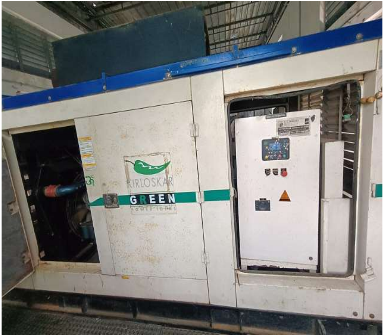
Fig.: 2.2- 250 KVA DG Set installed in college campus
