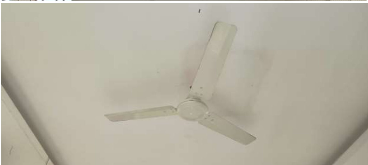
Fig.: 3.4 Electrical Equipments in Institute
