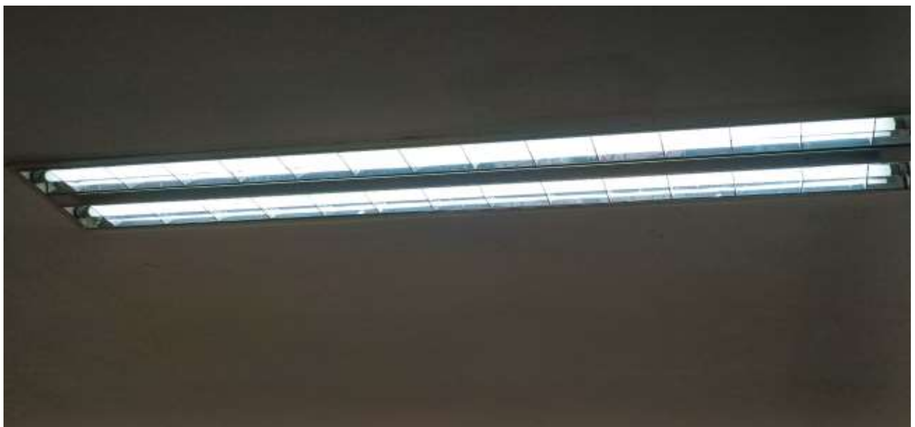
Fig.: 3.5 Electrical Equipments in Institute
