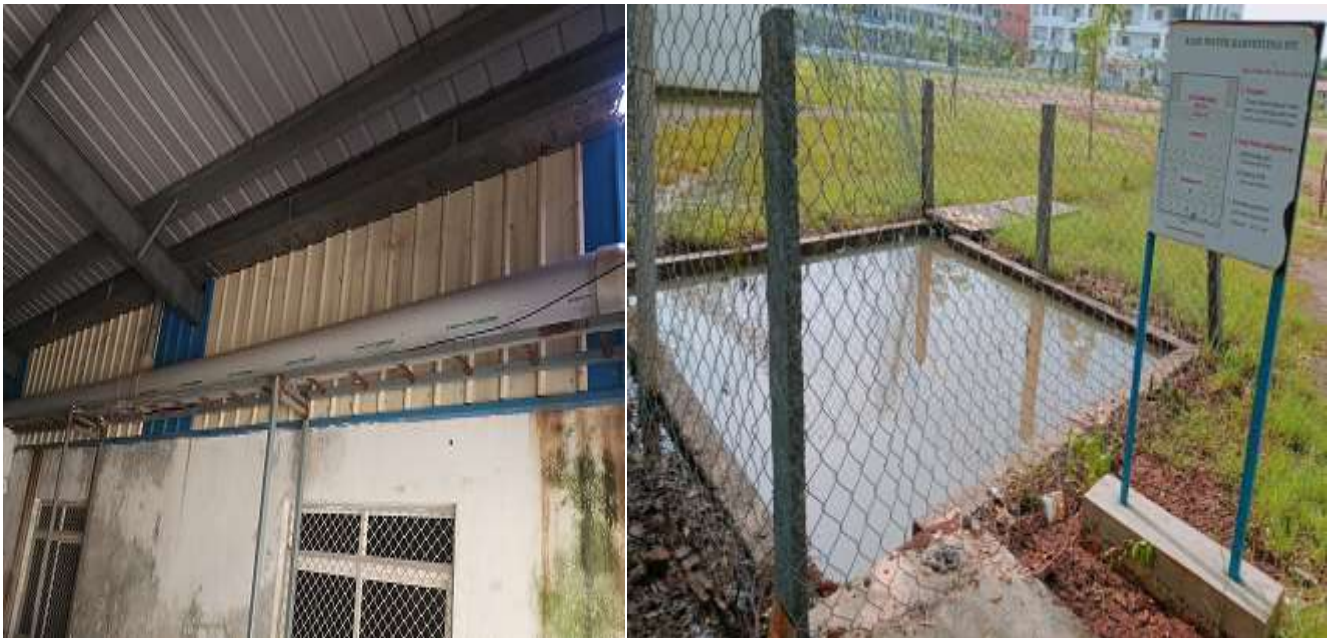
Fig.-3.2 Rain water collecting system of the institute
