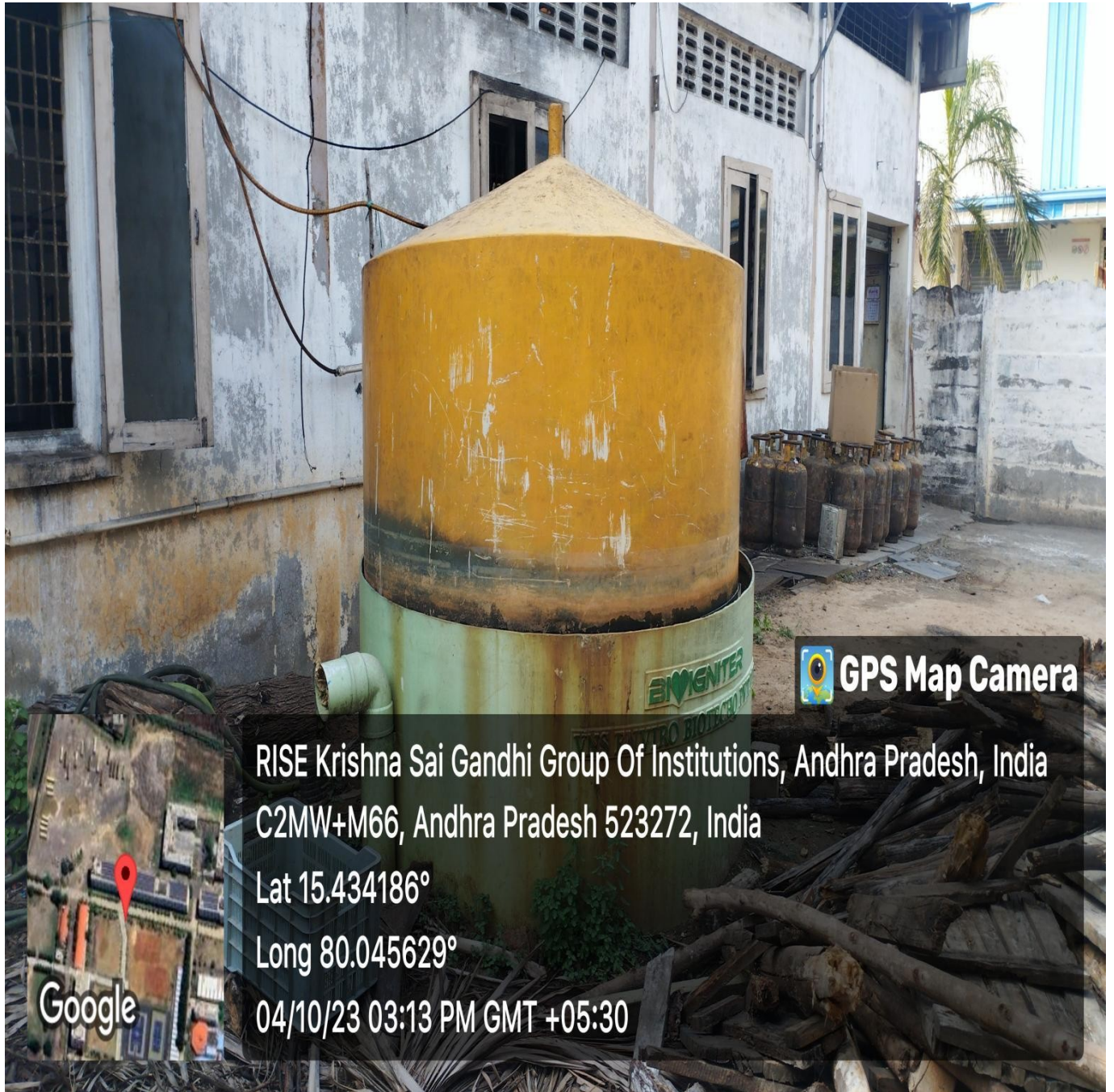
Bio gas PLANT
